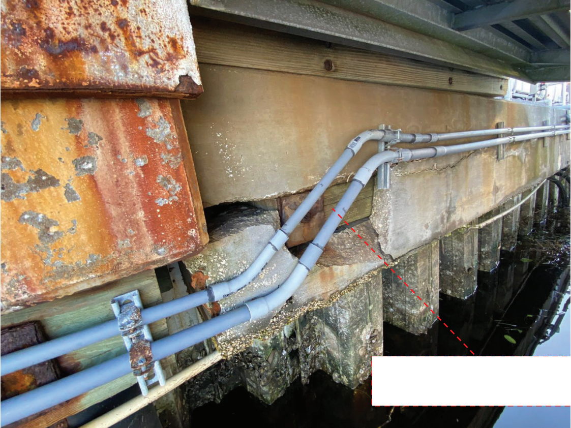
Photo #17 – View of Spalling in Wrap Cap.
