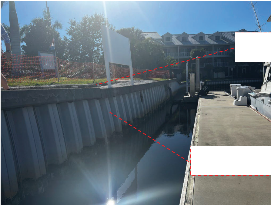
Photo #6 – View of Seawall Movement.
