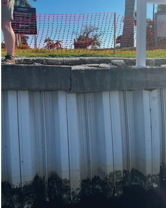
Photo #5 – View of Settling and Movement of Seawall.
